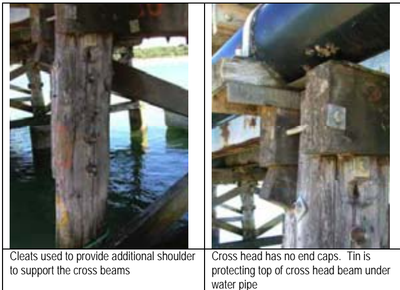
Photograph 2: Condition of crossheads
